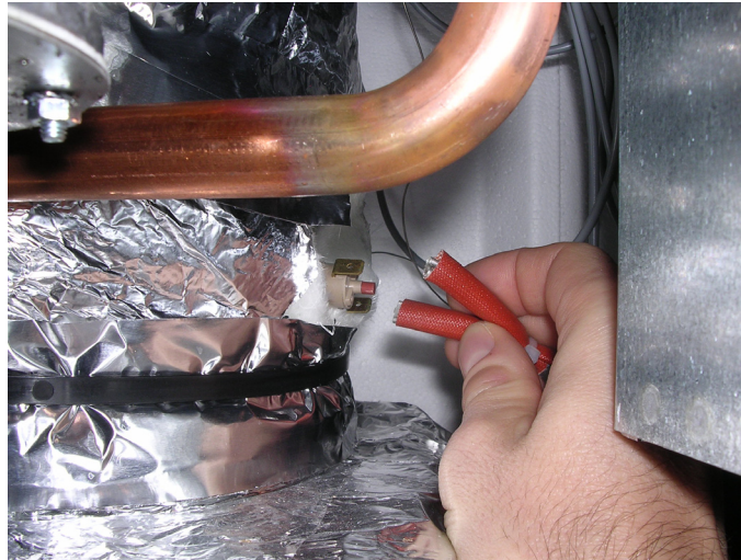
Figure 2 – Inspection at generator limit thermostat
